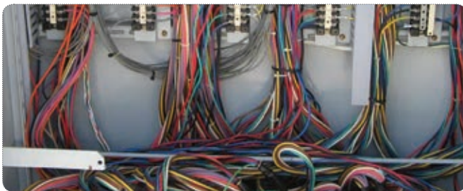
Many connections need to be made in each apparatus in the high voltage equipment switchyard
