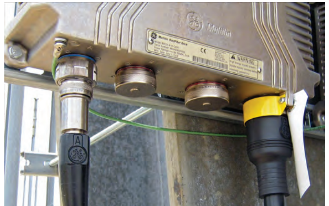
Figure 14. Safety device protecting against accidental opening of a live CT secondary circuit
