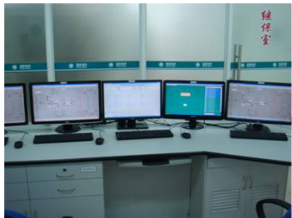
Figure 13 On site OWS photo
