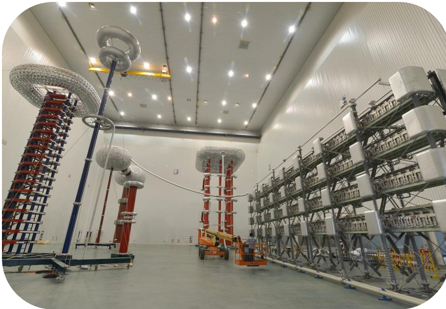
DC High Voltage Test
