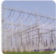
Highest AC Voltage Level 3 UHVAC 1000kV Substations
