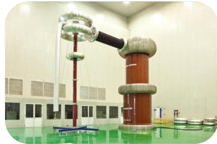
AC High Voltage Test
