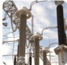
Over 100 110kV-750kV Lanxi Smart Substation
