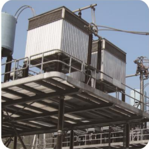
460 MVA & 540 MVA FSCs in 500kV Substations
