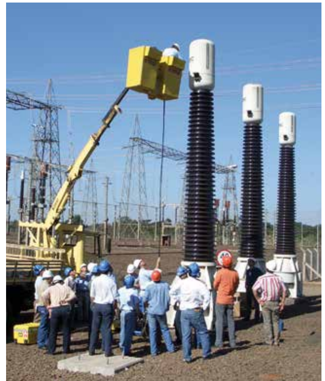
At the Itaipu dam, one of world's largest hydroelectric dams, the CPC 100 with CP TD1 was used for an impressive demo.
