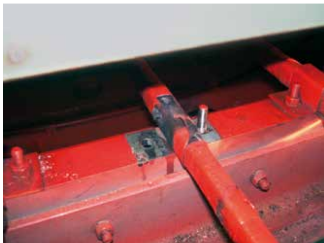
PD fault location on the output to the star point.
