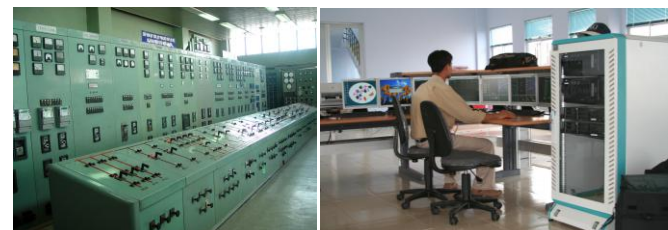
Fig. 6. Old and New Control Room Interfaces
