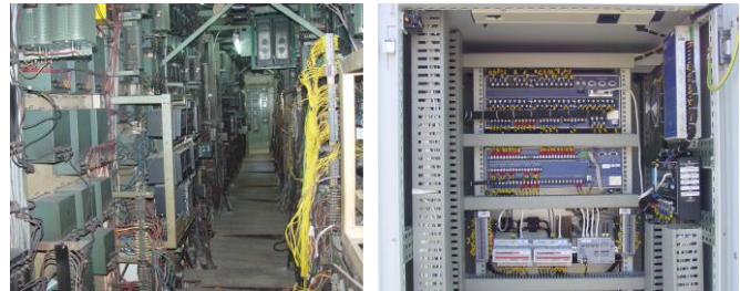
Fig. 4. Old and New Relay Panels
