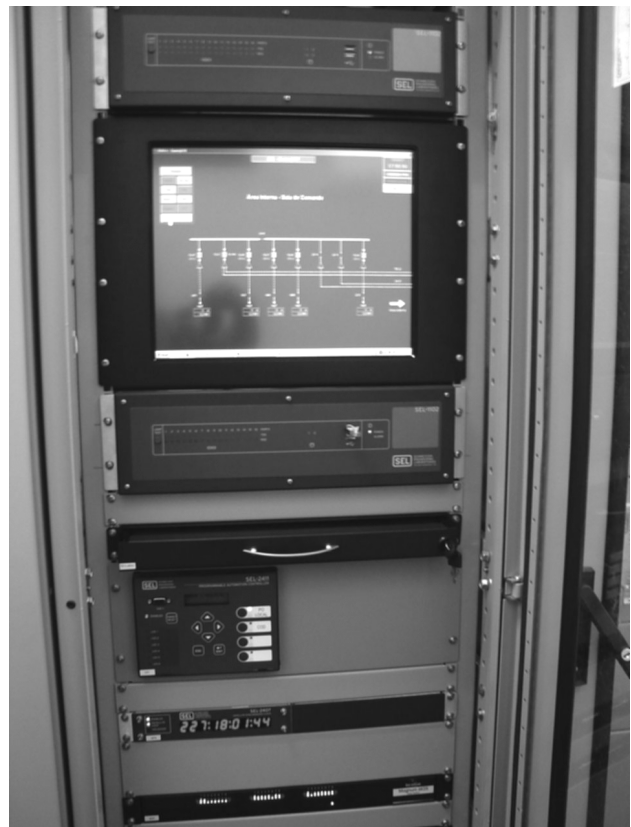
Fig. 7. Local HMI Panel
