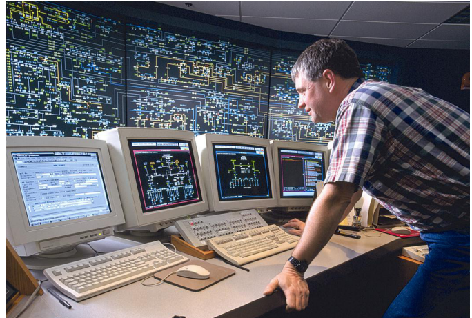
Fig. 3. Typical SCADA console user unaffected by choice of protocol within the substation
