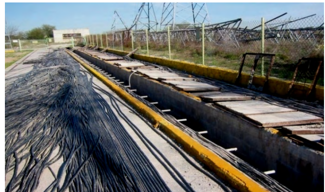
Fig. 3. Copper conductors removed from cable trenches and replaced by digital messaging.
