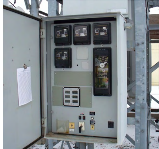
Fig. 3. Electromechanical relays in the yard
