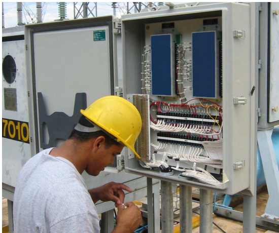
Fig. 5. I/O modules in the yard
