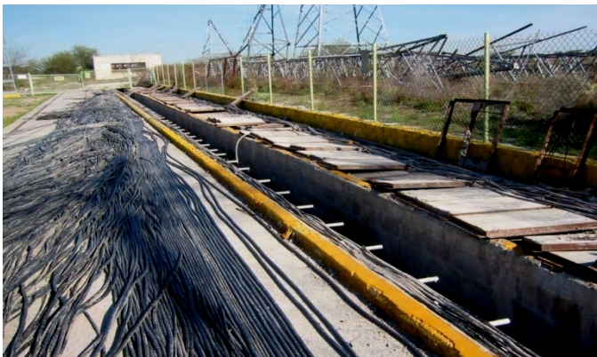
Fig. 6. Refurbishment project showing the amount of copper wire replaced with fiber-optic-based I/O module technology
