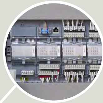
SICAM MIC installed in a separate RTU cubicle inside the transformer substation
